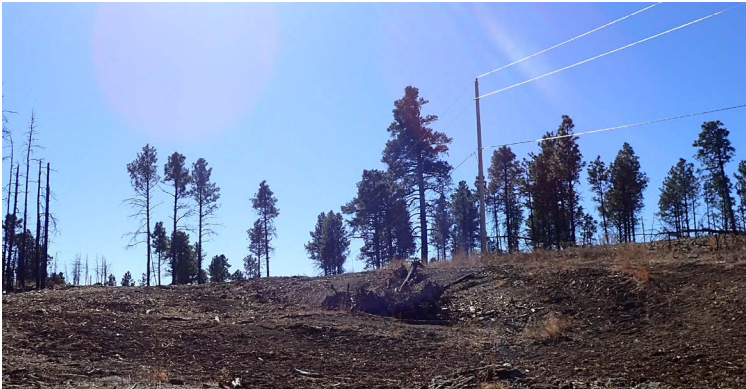
Tree hazard removal along the power line corridor created bare, compacted soil, lightly covered with masticated material.
