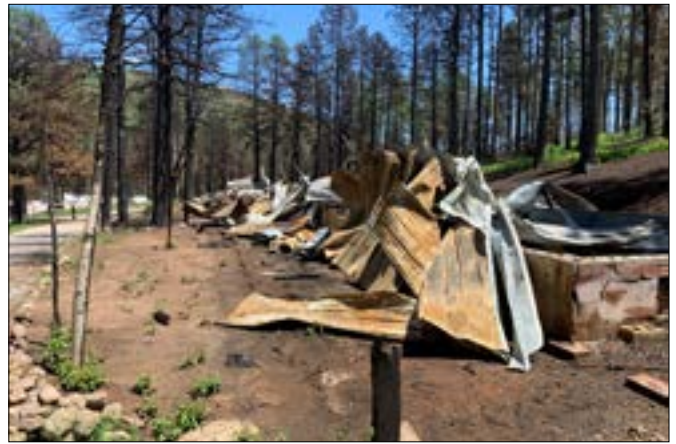
A burned building in the community of Pendaries, near Las Vegas, NM. Photo by Staci Matlock
