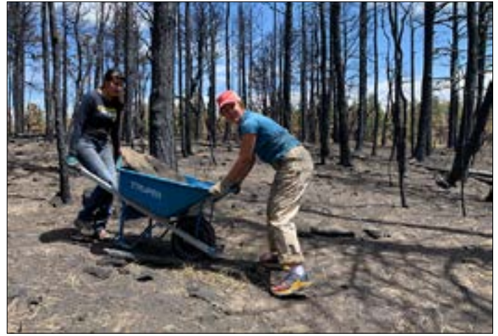
Natalia Shaw hauls rocks with NMFWR colleague Elliese Wright to build an erosion control structure. Photo by Staci Matlock.
