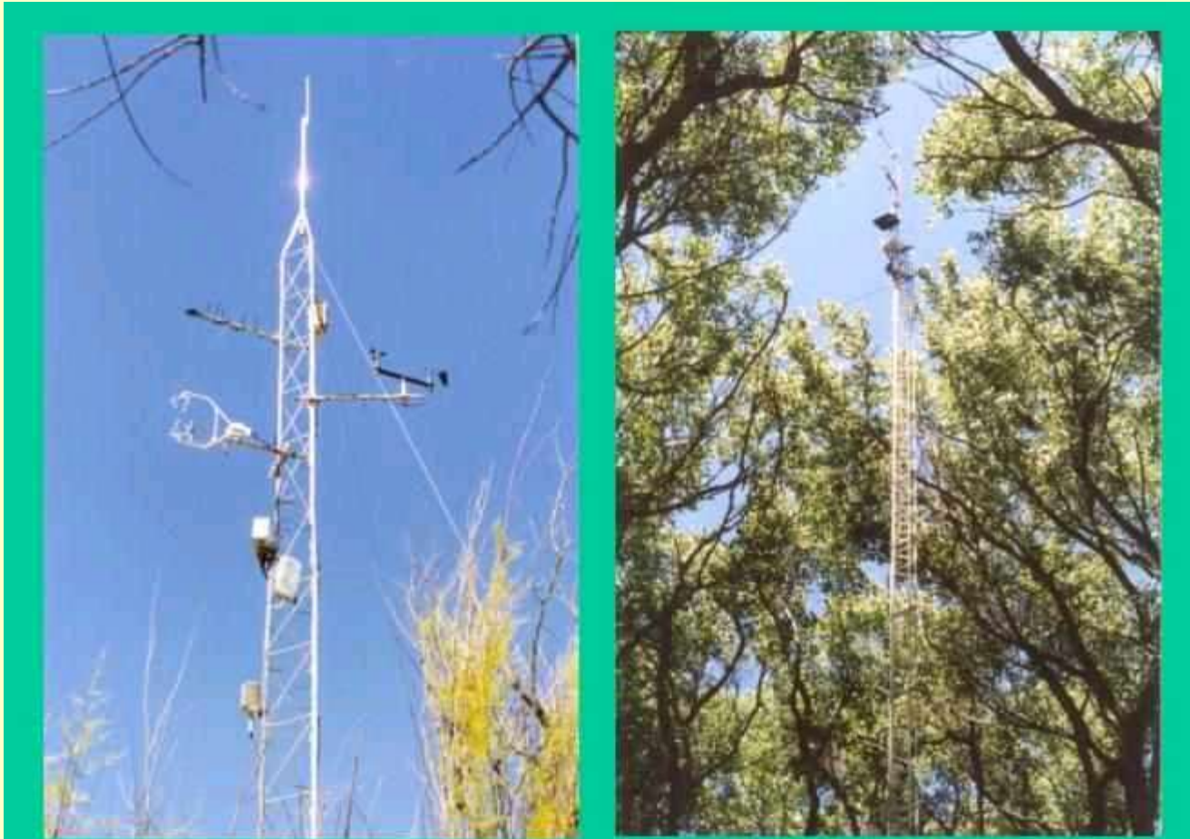
Figure 4. 10-m Tower in Salt Cedar Stand, 25-m Tower in Cottonwood Stand
