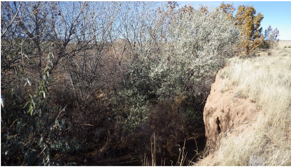
2015: SC5, view of San Cristobal drainage bend – cottonwood, Russian olive, and erosion. Taken facing 285 degrees.
