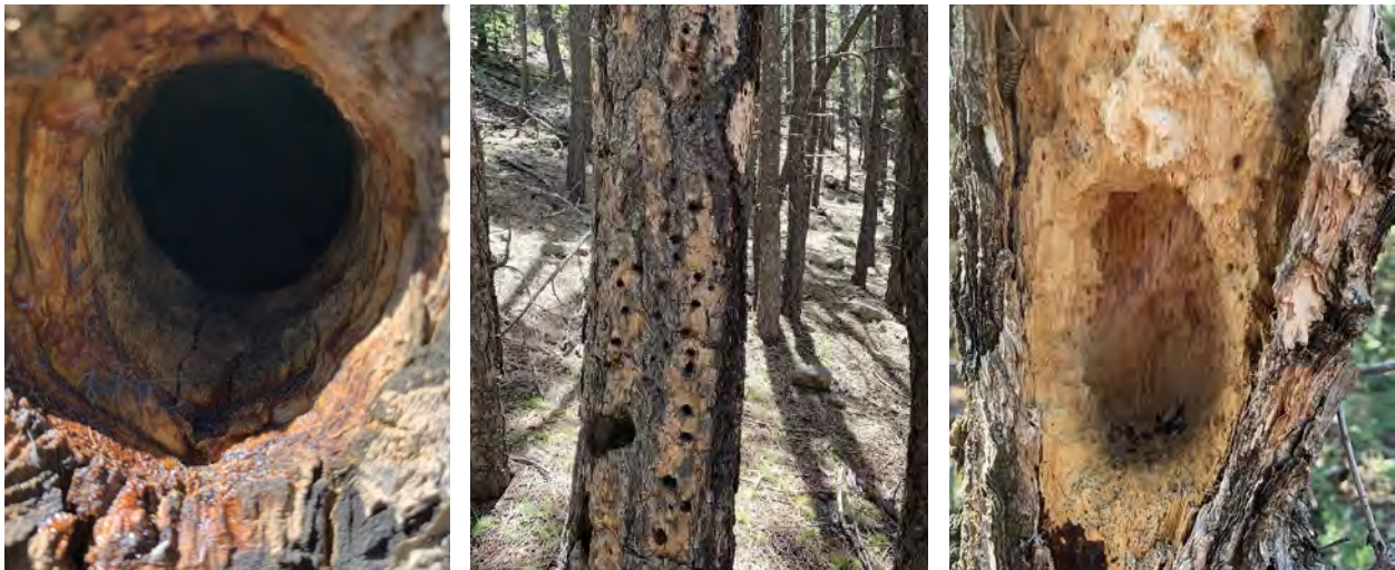
Damage caused by woodpecker (41010), note the deep irregular patterns of holes. Photos by Carmen Melendez
